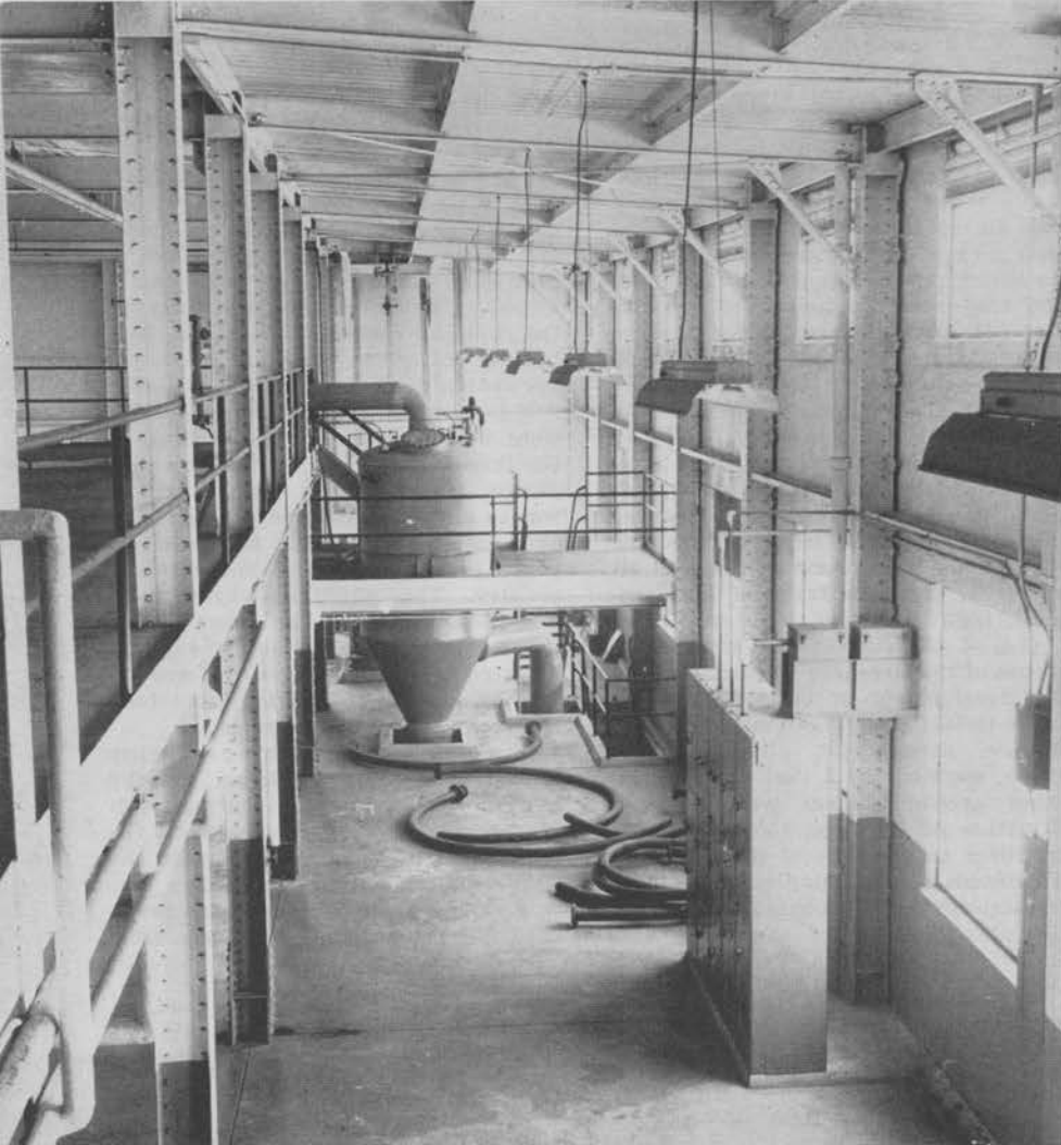
Inside the new Johnstown plant, a unique operation in the beet sugar industry. This view shows the top section of the MSG crystallizer. Many of the intricate facilities were engineered by GW personnel.
