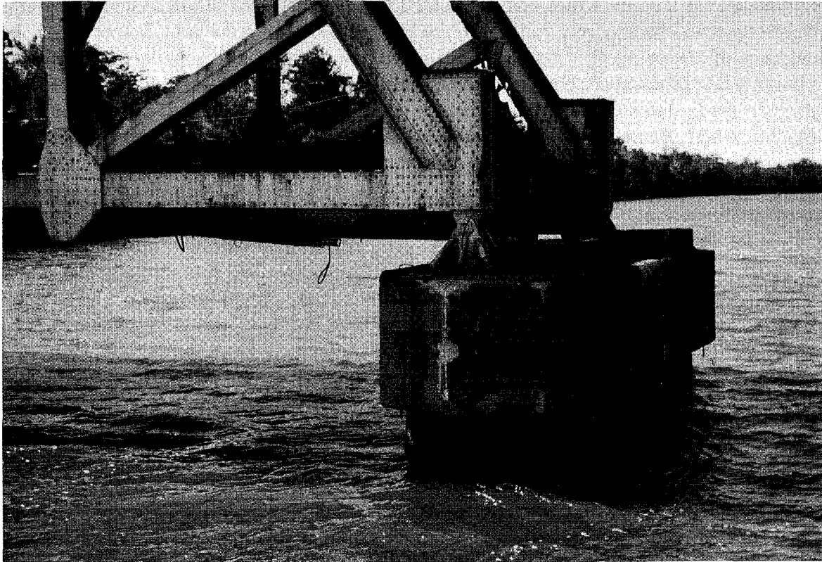
Figure 7.--Collision marks on Big Bayou Canot bridge.
